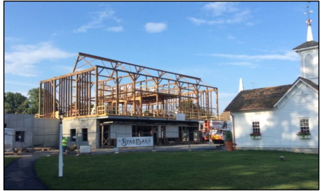
Image of Original Frame on New Site and Foundation with Relocated/ Rehabbed Outbuilding at Right. Photo: C. Leik.
