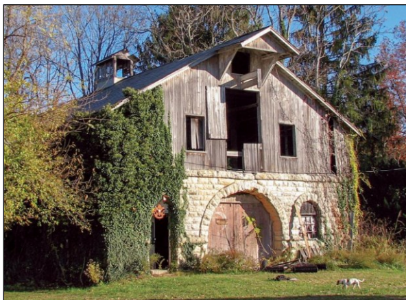
The foundation of the Cravenhurst barn is made of cut and dressed stones with arched entry to a central drive at the lower level. Photo credit: Indiana Landmarks. To learn more, visit: https://www.indianalandmarks.org/endangered-property/cravenhurst-barn/
