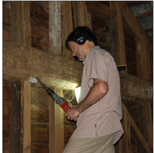
Dendrochronology requires core samples from the wood and must be taken from a waning edge, preferably with bark intact, of a structural member. Above is an image of a core sample being collected during this investigation. Photograph courtesy of Carla Cielo.
