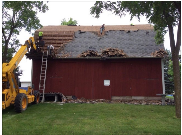
Above: View of workers removing asphalt-shingled roof and revealing original wood-shake roof underneath.
