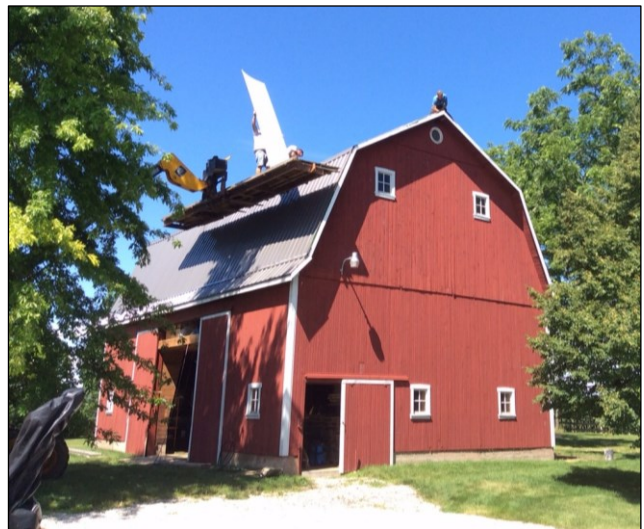
Below: View of roofers installing new steel sheeting on the Leik Family's circa-1936 barn.
