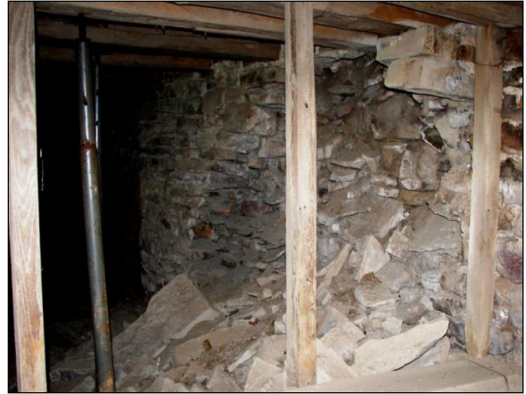
Interior Image of Typical Failure in Basement Wall of a Bank Barn
