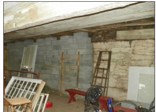
Interior Image of One Method for Repair: Construction of a New Cinderblock Wall to Support Failing Bank Wall Foundation
